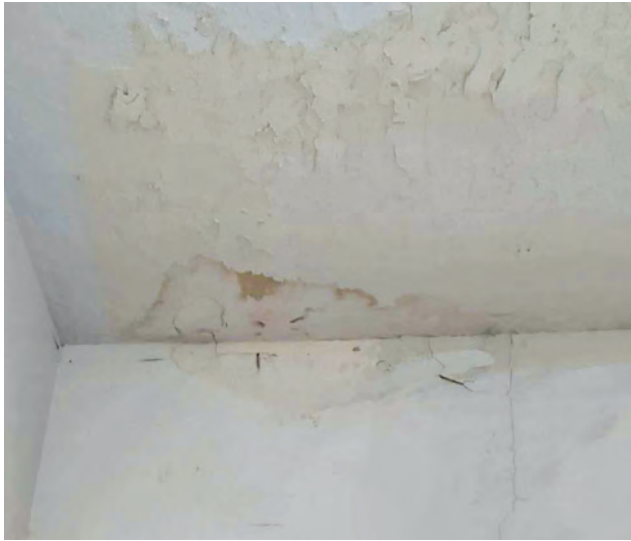
Evidence of water damage in a corner of one of the offices at the Grass Valley Community Center. File photo.
